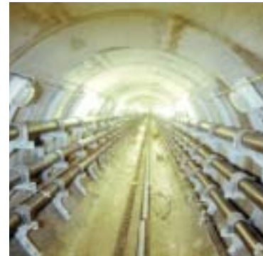
Internal view of high voltage underground cable tunnel.
